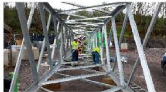
Cable sealing end tower assembly
