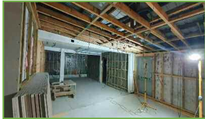
This was the area down the ramp where the freezers stood. This space will become the business and learning hub, with an entrance into the new toilets and a small kitchen for staff and volunteers.
