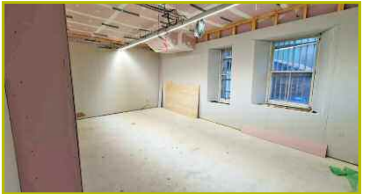
This is the storage area for the Reuse Shop. These windows were hidden behind the drink fridges. We have uncovered them to let light into this space.
